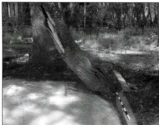
Figure 7. Northeast Corner of Foundation Showing Intrusion.
